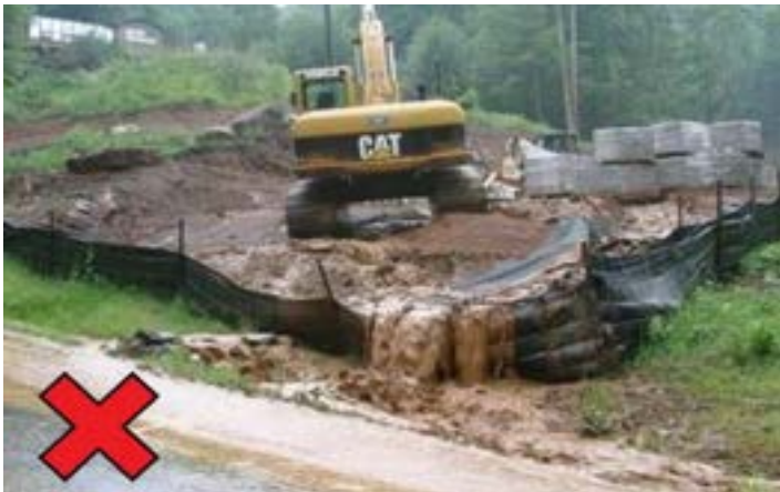
Figure 10: Silt fence failure
